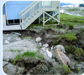
Moderating the Effects of Permafrost Degradation on Building Foundations
